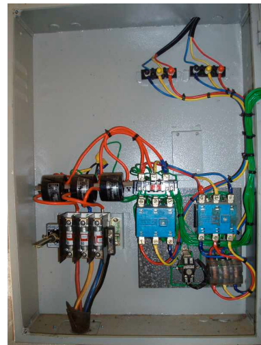
new control panel
