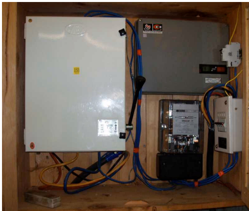
meter, main switch controls from the old pump
